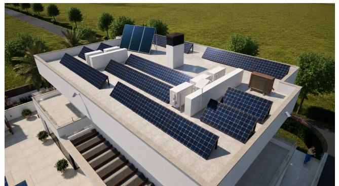
Roof with Airco's, Solar Panels, Heat Pump and Hot water Solar
